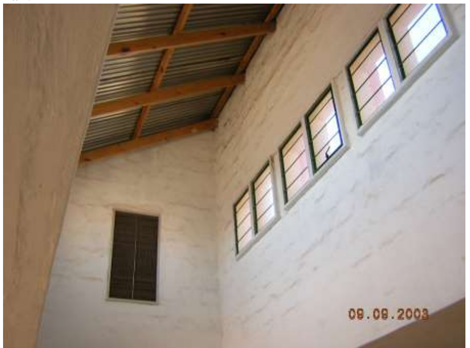
(Fig. 12); View up into the lantern from inside the main hall space.
